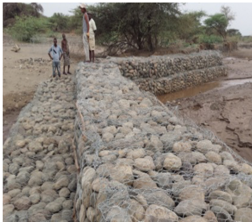
SSD river embankment protection work in Afar region. Source: SSD photo gallery
